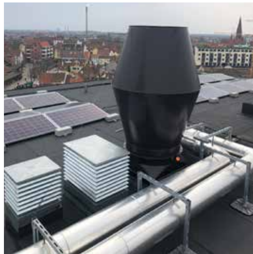
Air outlet from the kitchen
