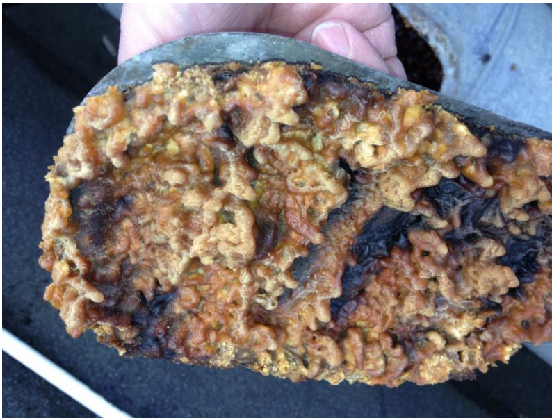
Grease deposit on inspection door
