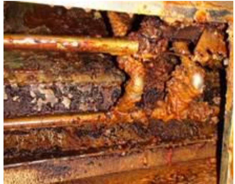
Grease deposits inside hood
