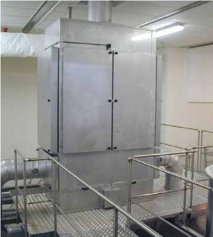
Air Treatment from two deep fat fryers. Total 8,000 m 3 /hr.
