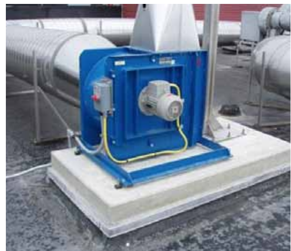
Fan placed on the roof.
