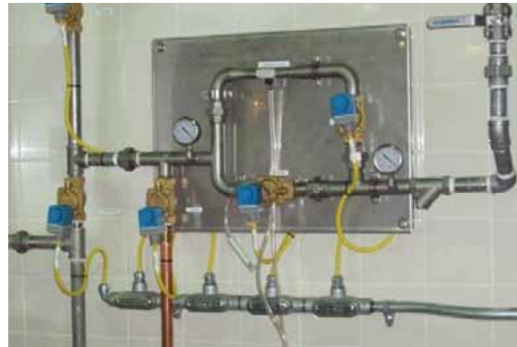
Automatic cleaning system.
