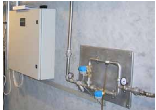
Control Board Automatic CIP cleaning unit.
